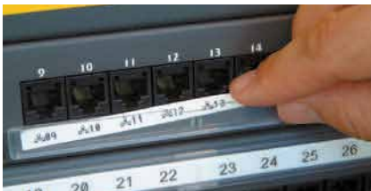
Punch Block & Patch Panel Labels
