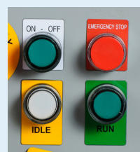
Control panel labelling
