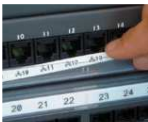
Punch block & patch panel labels
